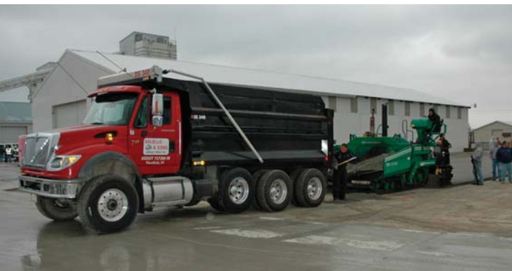
The light-duty pavement serves a parking area for the Concrete Store, stocking decorative flatwork tools and finishing products.
