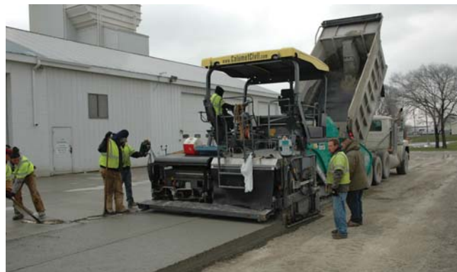
The heavy-duty RCC slab links a perimeter and central truck path at Builder's Concrete's Fishers, Ind., headquarters operation.
